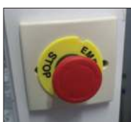
Emergency stop button
