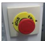
Emergency stop button
